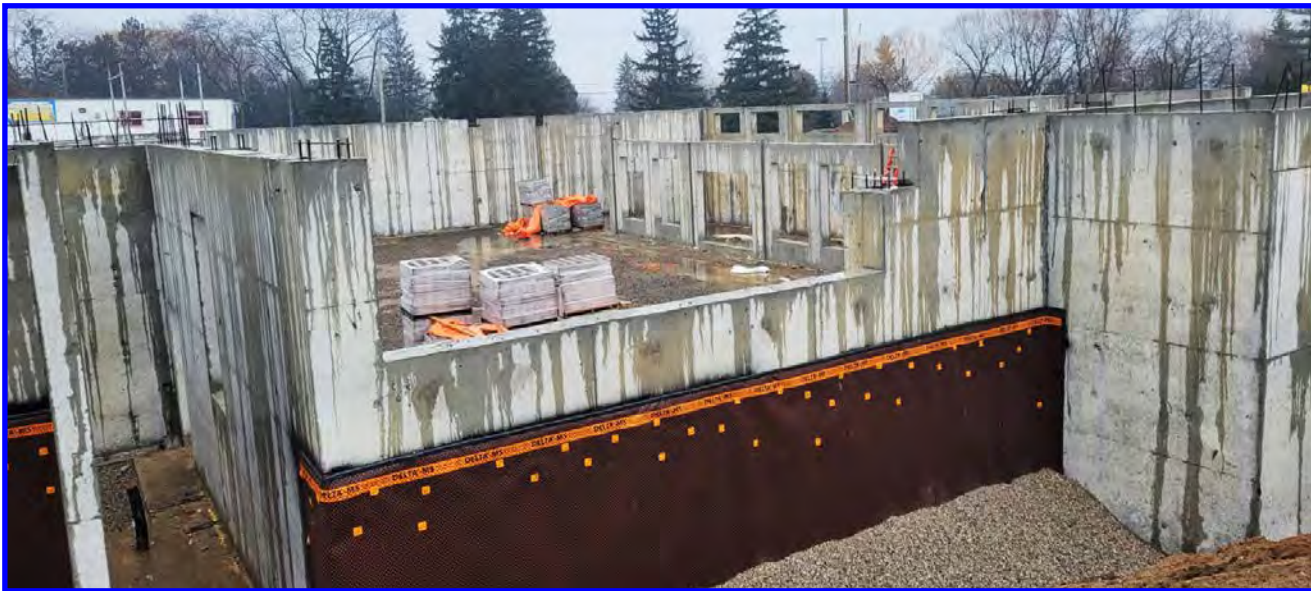
With its walls completed, Radha Krishna Mandir is starting to show its serenity & presence
